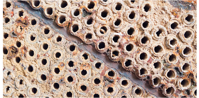
Scaling on heat exchanger tubes
